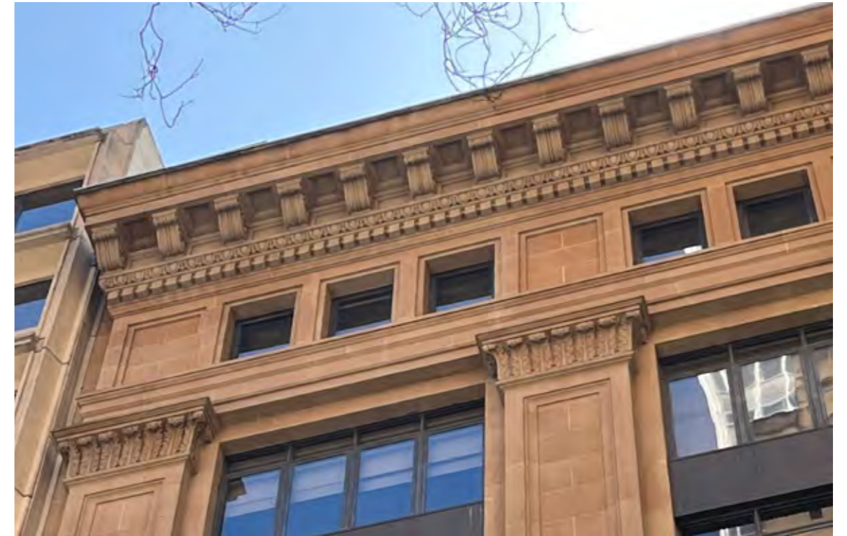
Decorative top cornice has considerable depth and is prominent within O'Connell Street. Image source: Stewart Architecture
